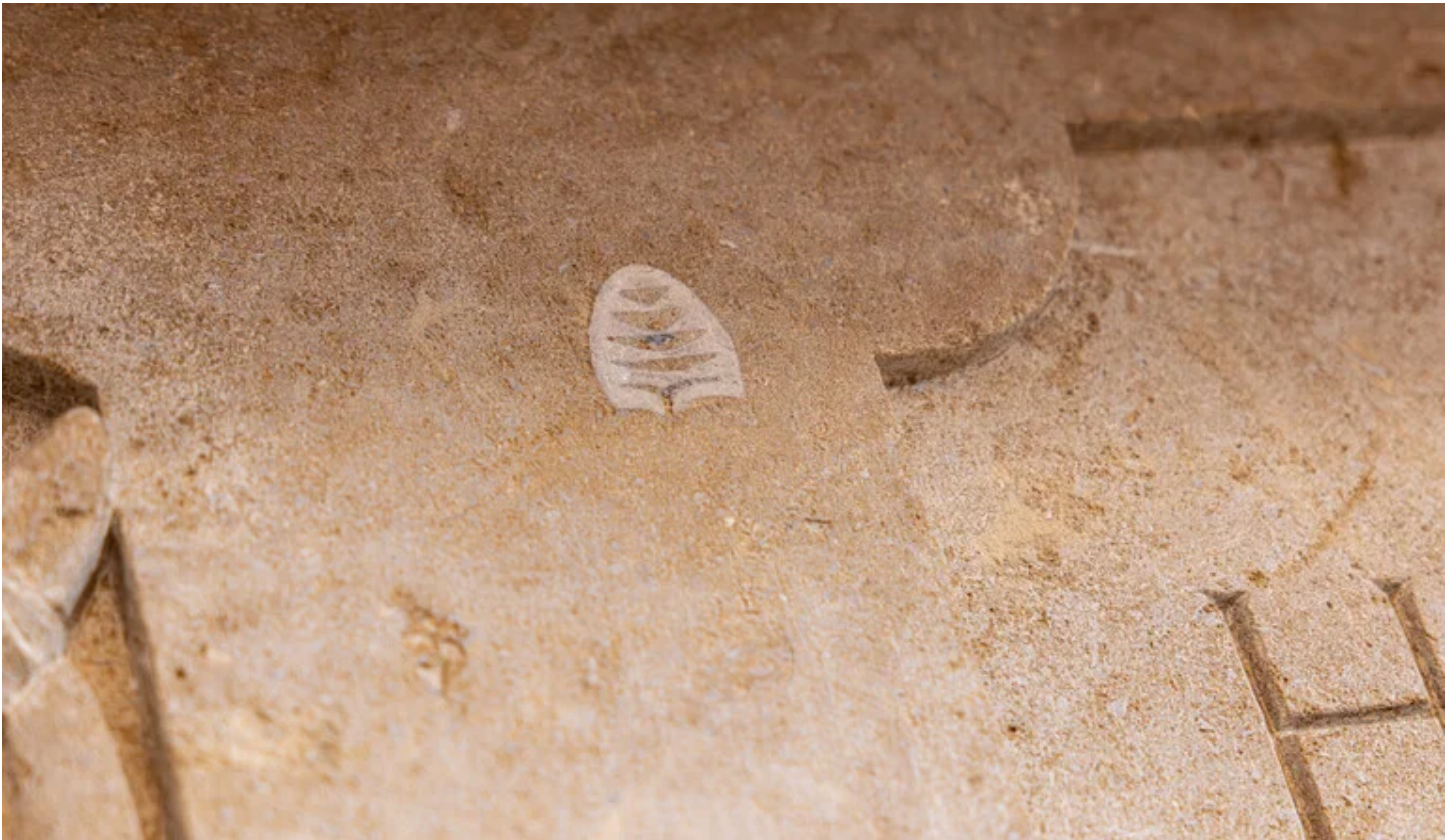
The great stone and brick fireplace was cleaned, revealing small fossils embedded in the stone.
